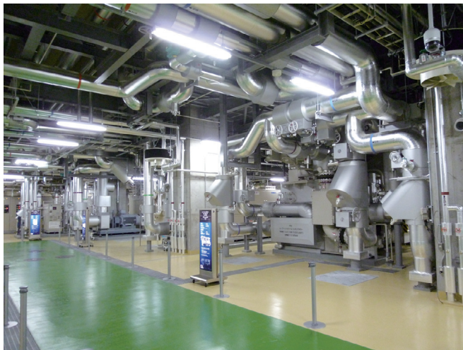
Main plant of DHC system
