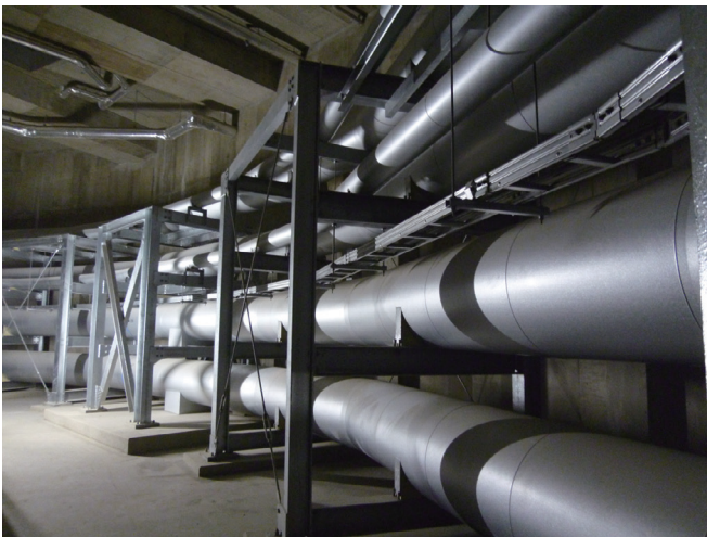
Pipes circulating in the DHC supply district
