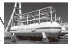
Ammonia Storage Tank
