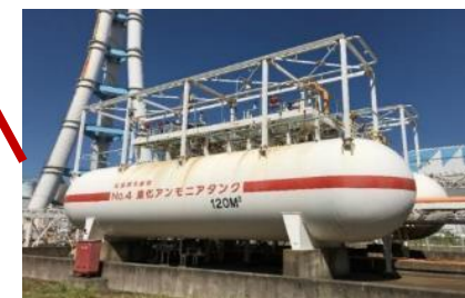
Ammonia Storage Tank
